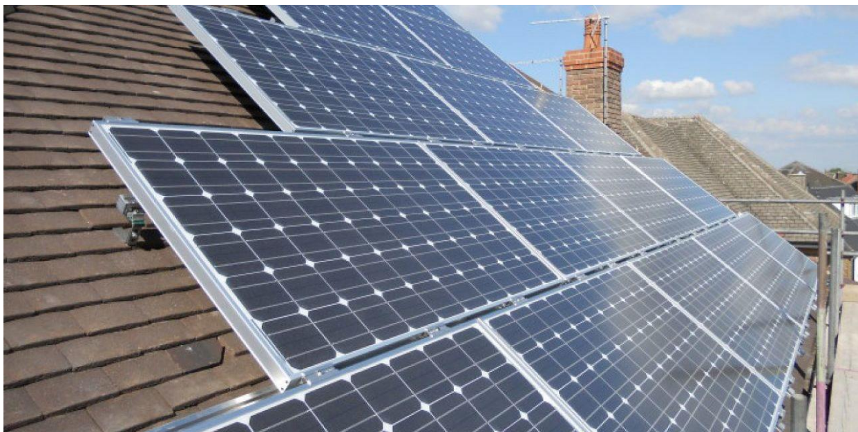
Figure 32: Micro PV installation
